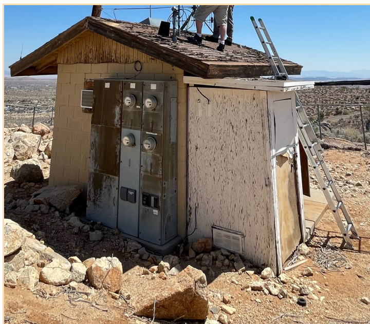
A file photo from before the roof replacement, showing the "eyesore" shed still begging removal. – Photo by N6GKB
