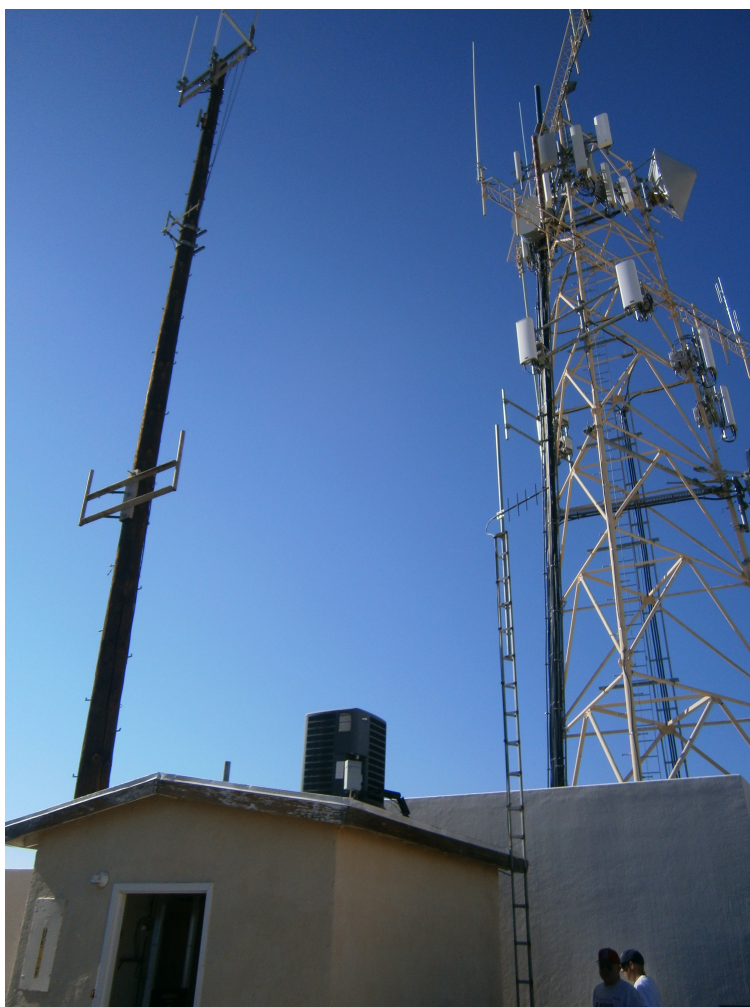
The repeater antenna is atop the wooden pole on the left. The repeater building in foreground. – Photo by Larry AD6G
