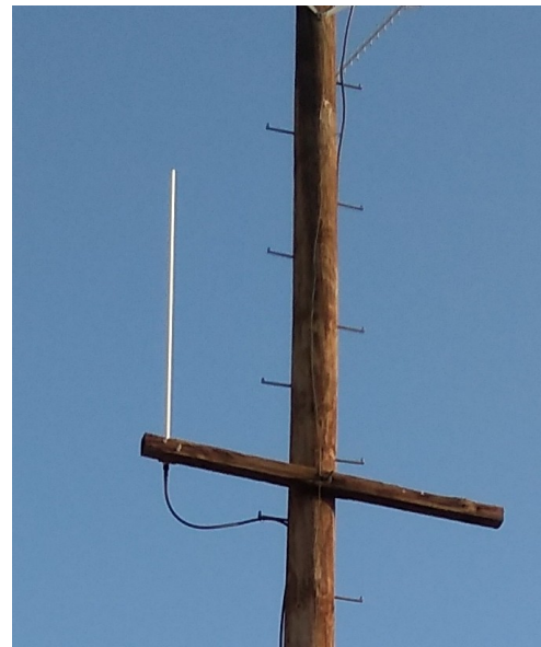
New antenna connected to hardline. — Photo by AD6G
