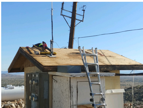
The roof is nearly prepared for the new shingles. — Photo by N6GKB
